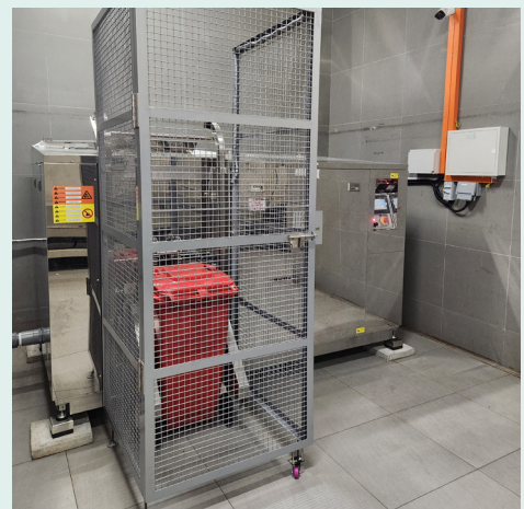
Food waste biodigester installed at Funan which commenced its pilot in late 2022
